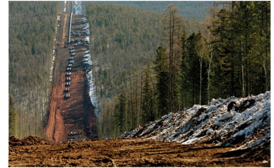
The Power of Siberia gas pipeline takes natural gas from Irkutsk, Russia, to the far east of the country and China.
